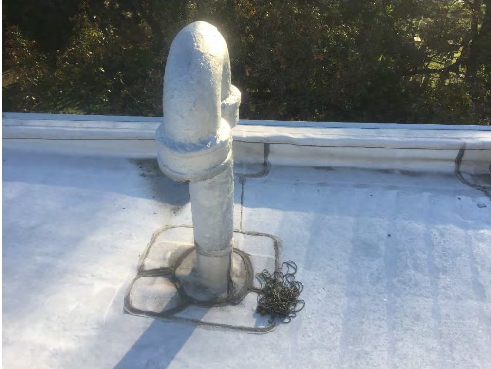
Drain Exhaust Vent
