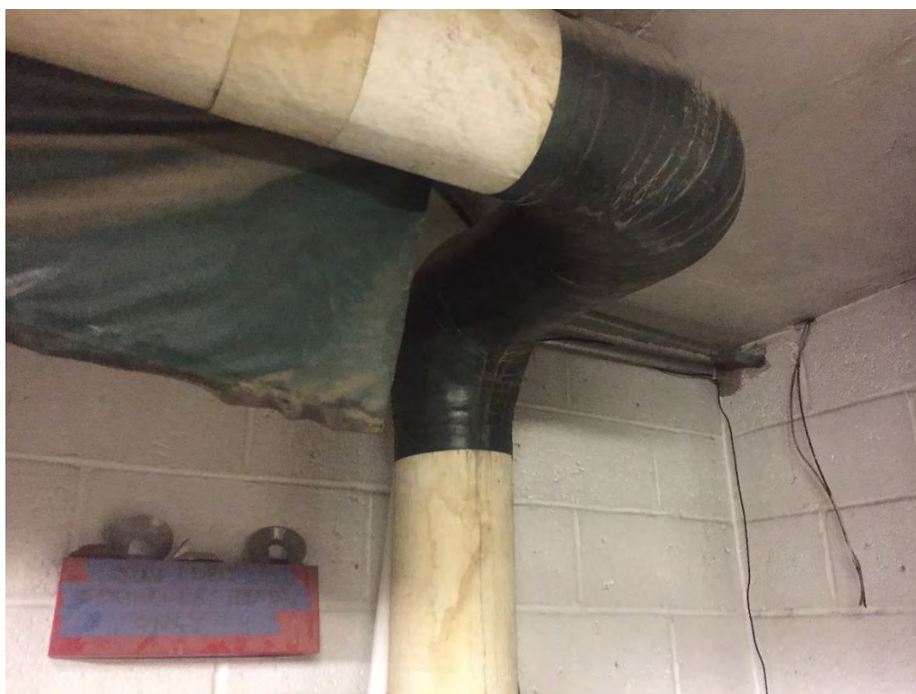
Sprinkler Room Fittings
