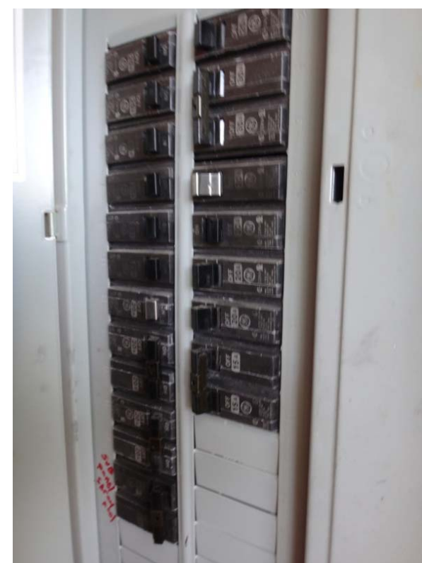
PHOTO C - PANEL LP Existing Utility Room Panel In Field House With Space For New Lighting
