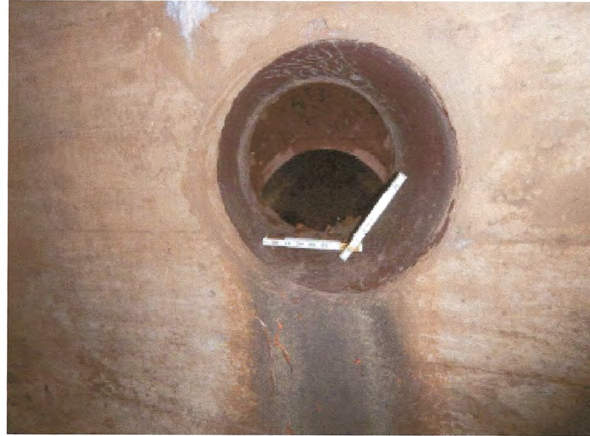
PICTURE LOCATION: SOUTH END OF THE WEST SIDEWALK, MISALIGNED DRAINAGE PIPE AND EXPOSED FILL
