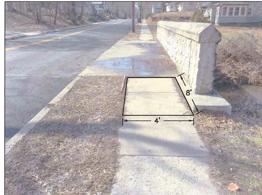
LOCATION 15.B LIMIT OF SIDEWALK REPLACEMENT TO SOUTHWEST APPROACH SIDEWALK - 4 SQUARE YARDS
