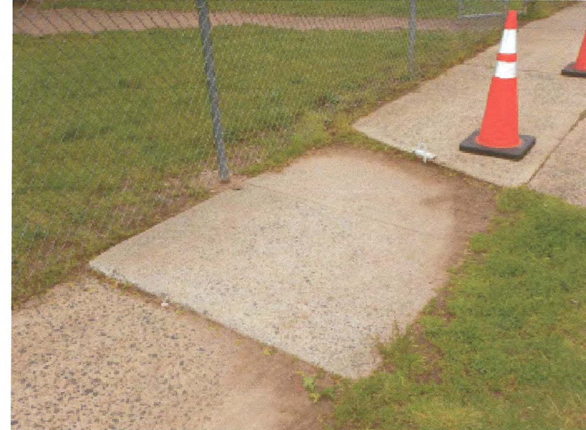
PICTURE LOCATION: SOUTHEAST APPROACH SIDEWALK, LOOKING SOUTHWEST. SETTLEMENT OF UP TO 2"
