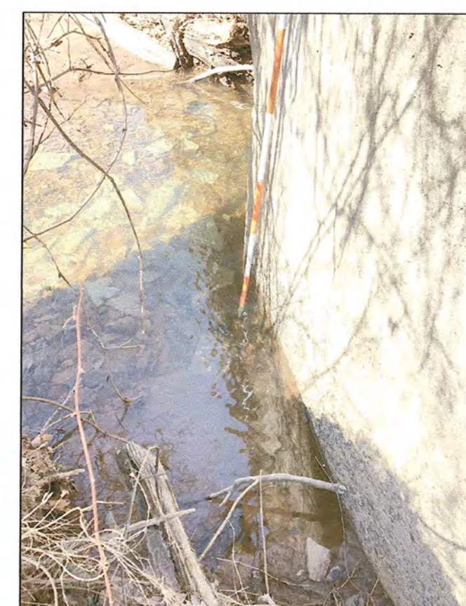
PICTURE LOCATION: SOUTHWEST WINGWALL, LOOKING NORTH. SEVERE EROSION IS PRESENT
