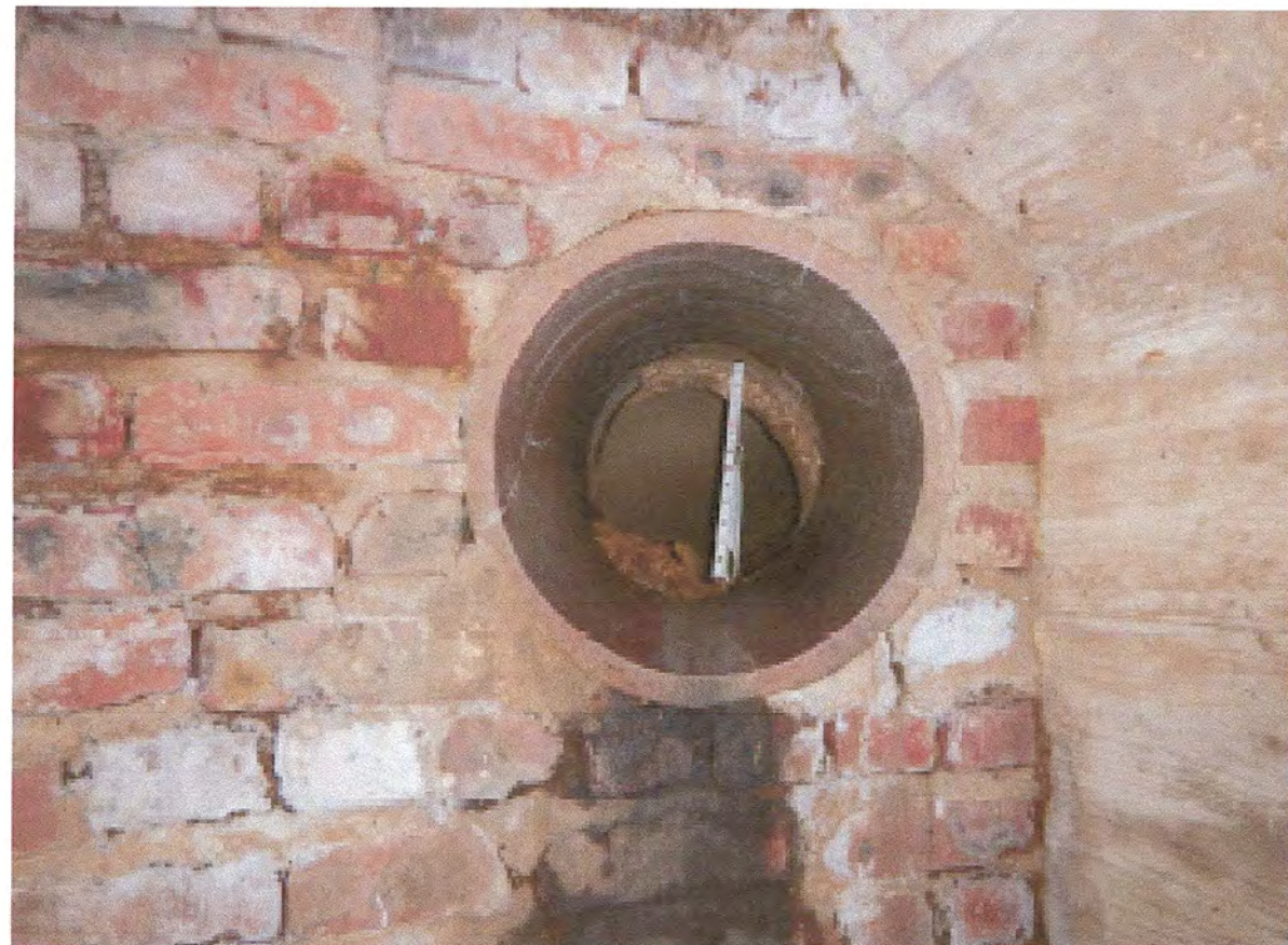
PICTURE LOCATION: BRICK MASONRY WALL AT THE NORTH END OF THE CULVERT, LOOKING NORTH. PIPE MISALIGNMENT WITH EXPOSED FILL.
