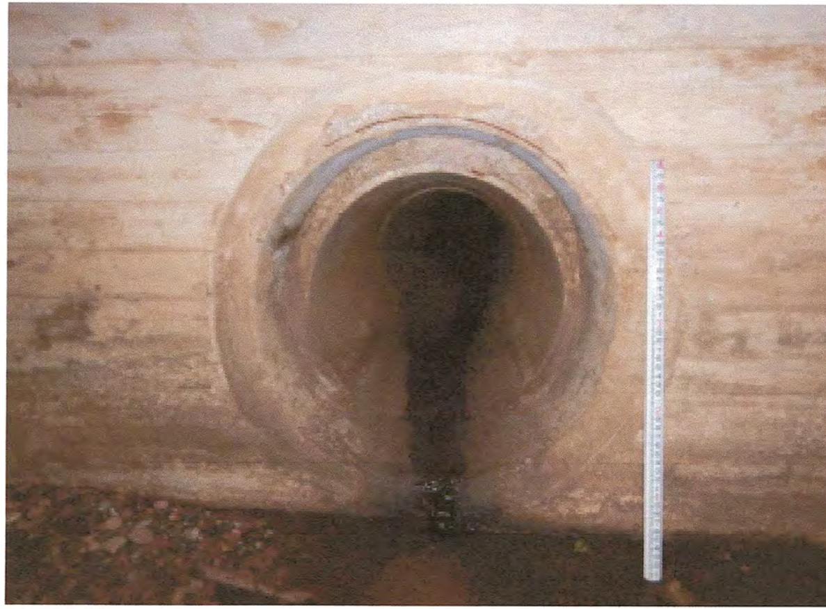
PICTURE LOCATION: EAST ABUTMENT DRAIN OUTLET PIPE AT NORTH END, LOOKING EAST. SPALL WITH EXPOSED REINFORCEMENT.
