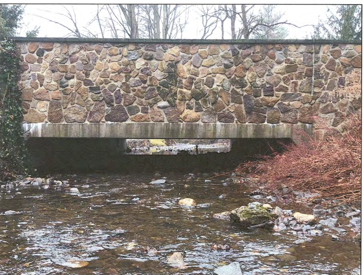
PICTURE LOCATION: TAKEN UPSTREAM FACING DOWNSTREAM WHERE DEBRIS BUILDS UP AT UTILITY PIPE CROSSING.
