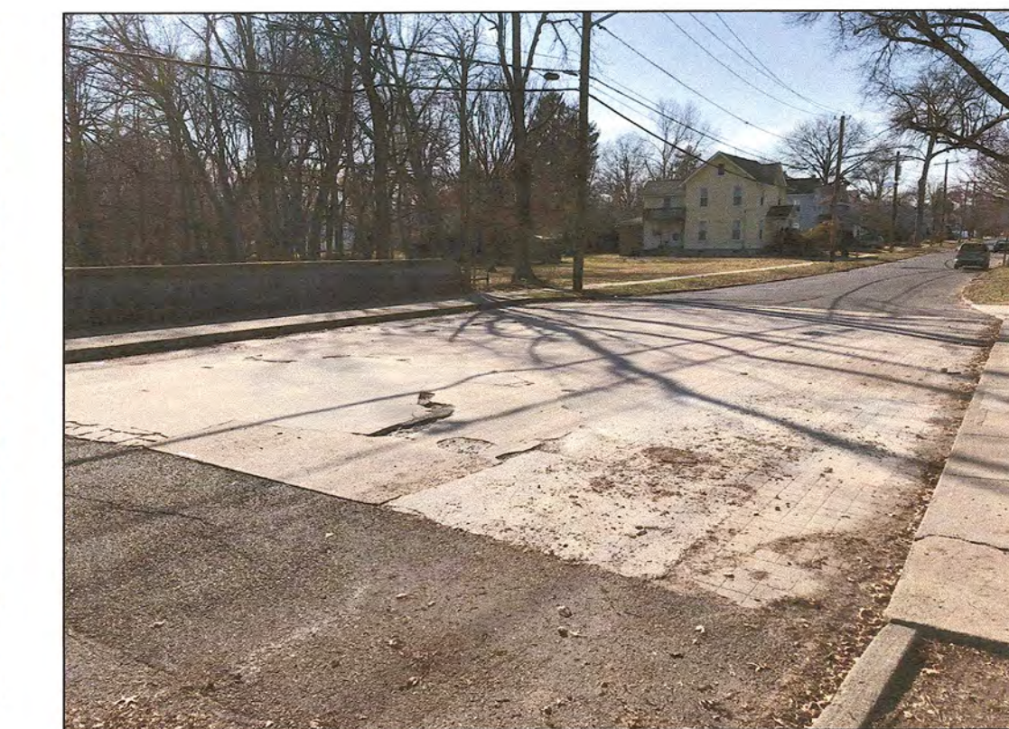
LOCATION 22: NORTHEAST APPROACH SIDEWALK, LOOKING SOUTHWEST. THE DECK IS HEAVY SPALLED AND DELAMINATED.
