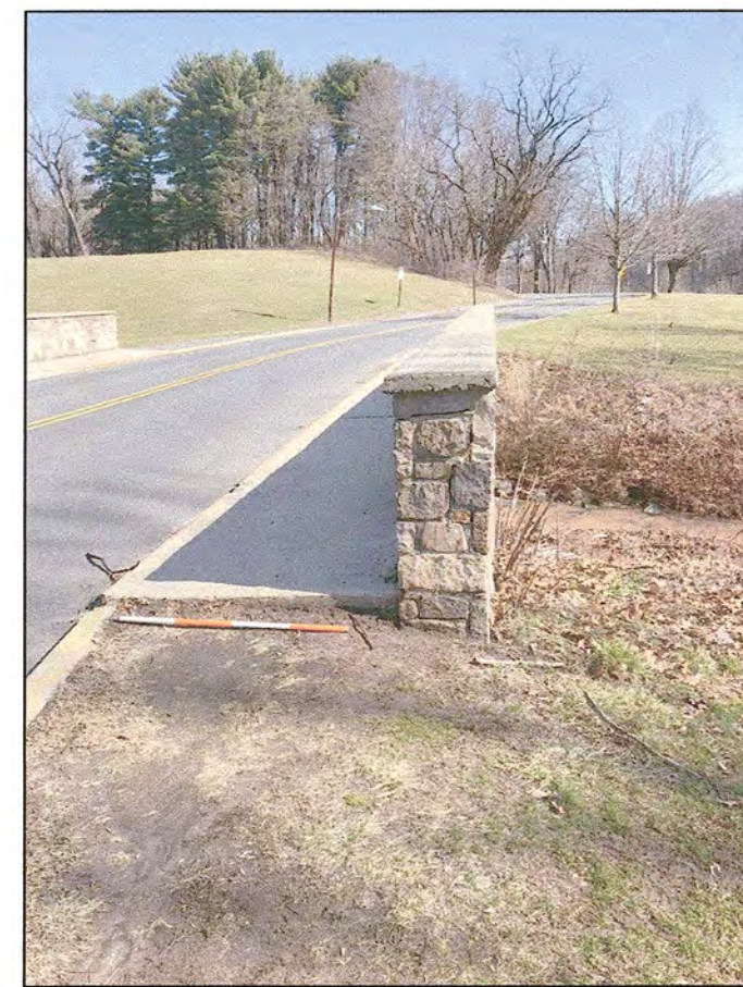
PICTURE LOCATION: SOUTHWEST BRIDGE APPROACH, LOOKING EAST. THERE IS EXPOSED SIDEWALK PRESENTING A TRIPPING HAZARD
