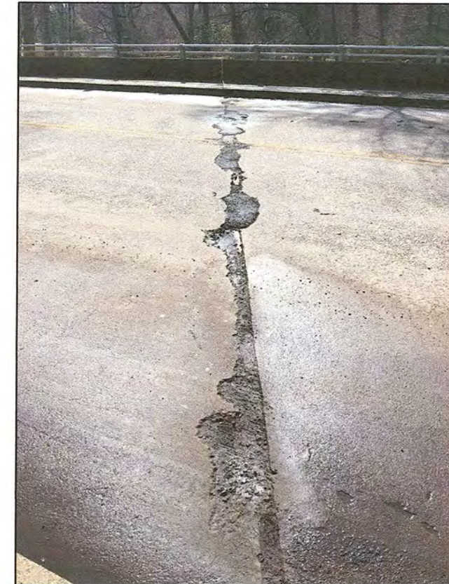
PICTURE LOCATION: MIDDLE JOINT, LOOKING EAST. SPALLS TYPICAL THROUGHOUT
