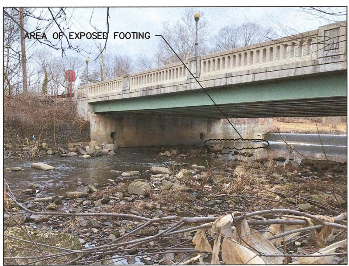
PICTURE LOCATION: SOUTH ELEVATION, LOOKING NORTH. (BACKGROUND) THE WEST RETAINING WALL EXHIBITS AREAS OF EXPOSED FOOTINGS.
