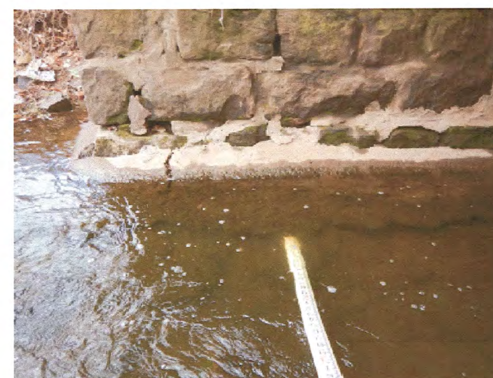
LOCATION 22: SOUTH END OF WEST ABUTMENT, LOOKING WEST. UNDERMINING BELOW THE CONCRETE SCOUR PROTECTION
