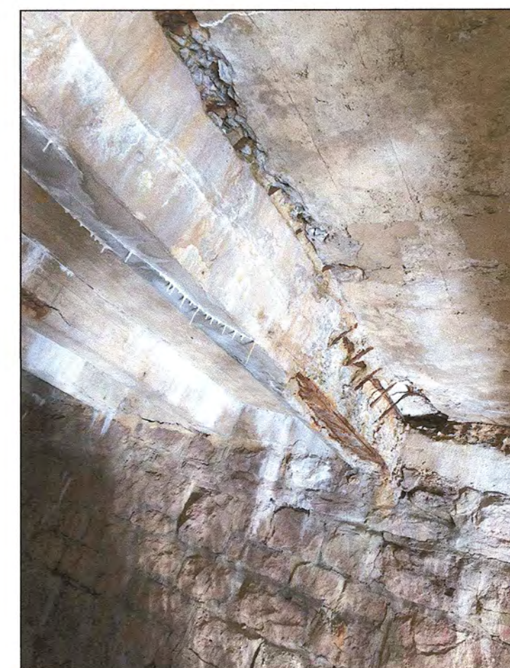
LOCATION 22: EAST SPAN UNDERDECK, LOOKING EAST. HEAVY SPALLING WITH EXPOSED REINFORCEMENT IN DECK AND BEAMS
