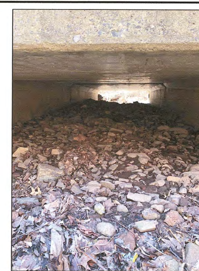
PICTURE LOCATION: NORTH CELL, LOOKING EAST. THE NORTH CELL IS HEAVILY BLOCKED
