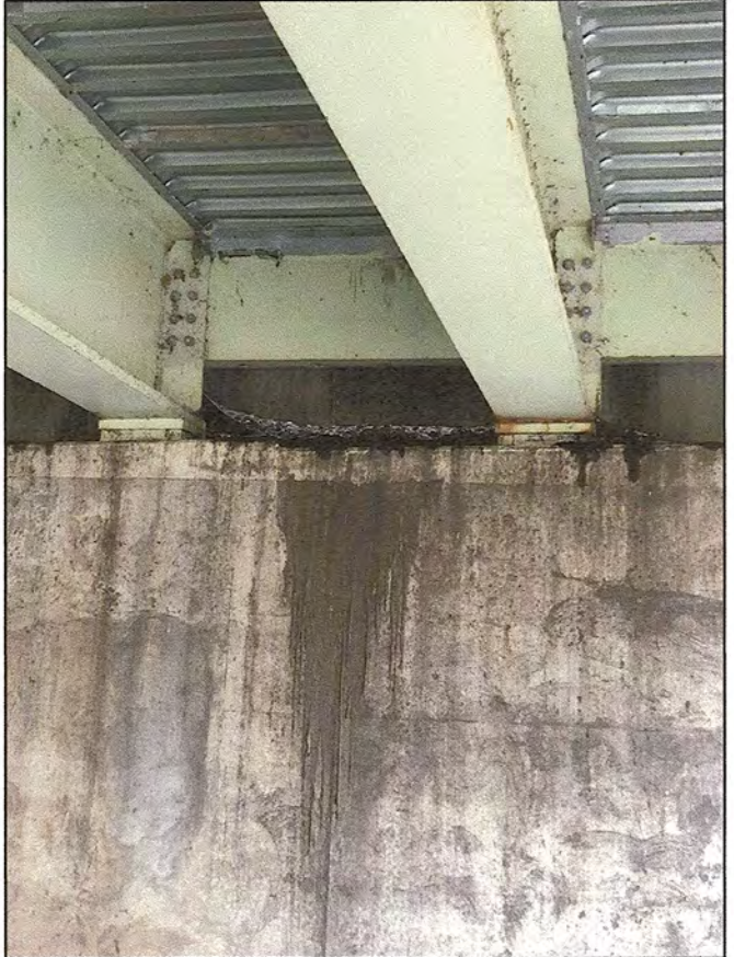
PICTURE LOCATION: EAST ABUTMENT, LOOKING EAST. SUNKEN JOINT MATERIAL RESTING ON ABUTMENT BREASTWALL
