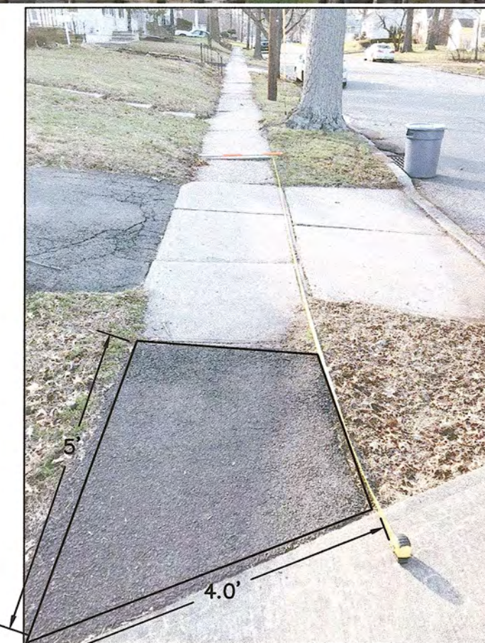
PICTURE LOCATION: SOUTHWEST APPROACH SIDEWALK, LOOKING WEST. THE BITUMINOUS SIDEWALK IS DEPRESSED
