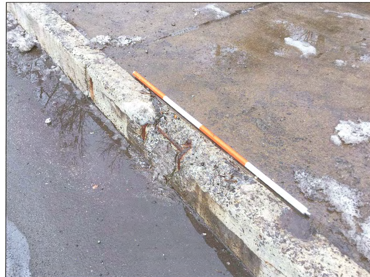
LOCATION 20: SOUTH BRIDGE CURB, LOOKING SOUTHEAST. THERE IS SEVERE SPALLING AND EXPOSED REINFORCEMENT FOR APPROXIMATELY 25 LF
