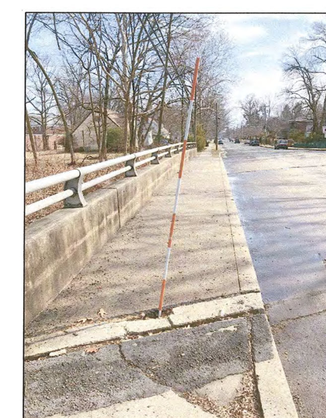
BRIDGE HEADER AT NORTHWEST APPROACH SIDEWALK. THE HEADER IS DAMAGED
