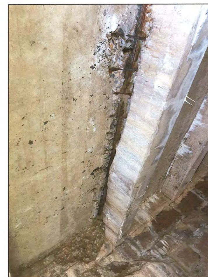
LOCATION 22: WEST SPAN UNDERDECK, LOOKING WEST. HEAVY SPALLING WITH EXPOSED REINFORCEMENT IN DECK AND BEAMS
