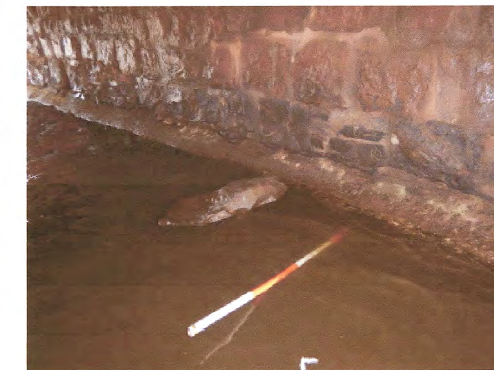
LOCATION 22: WEST FACE OF CENTER PIER, LOOKING NORTHEAST. UNDERMINING BELOW THE CONCRETE SCOUR PROTECTION
