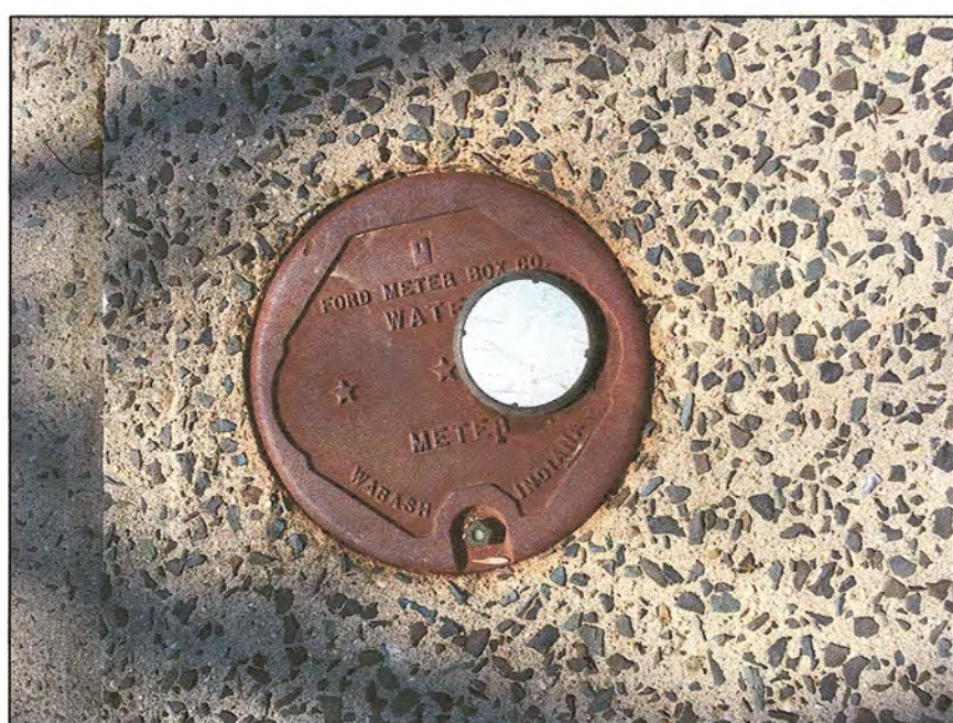
IMAGE SHOWS WATER METER LOCATED WITHIN SIDEWALK EXTENTS TO BE REPLACED.
