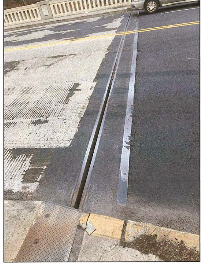
PICTURE LOCATION: EAST ABUTMENT JOINT, LOOKING NORTH. THE JOINT MATERIAL HAS FAILED
