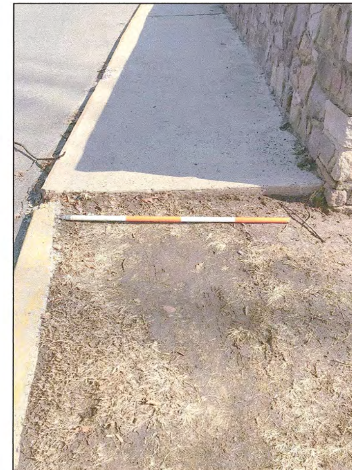
PICTURE LOCATION: SOUTHWEST BRIDGE APPROACH, LOOKING EAST. THERE IS EXPOSED SIDEWALK PRESENTING A TRIPPING HAZARD
