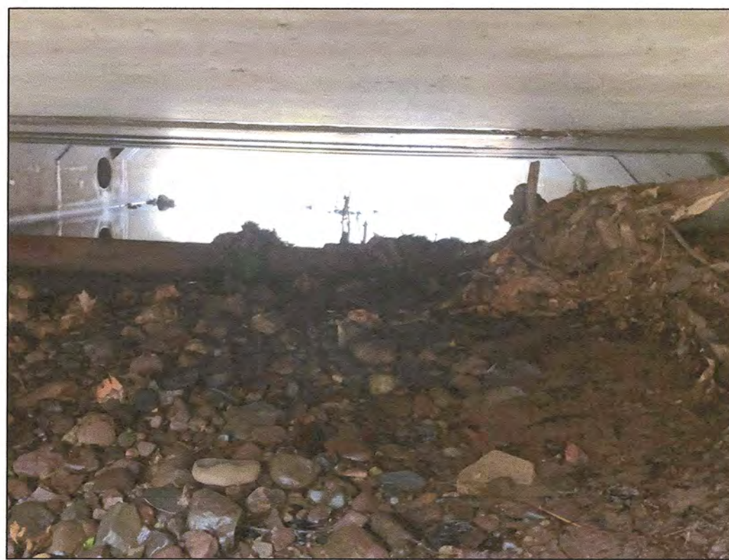
IMAGE SHOWS THE DEBRIS BUILD UP LOOKING EAST (DOWN STREAM) AT THE NORTHERN ABUTMENT.
