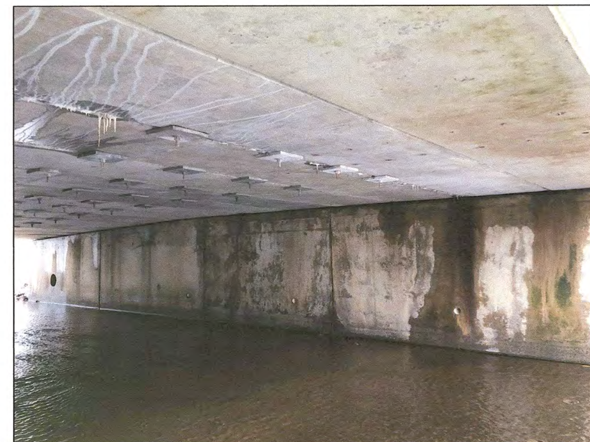
PICTURE LOCATION: SOUTH BRIDGE ABUTMENT, LOOKING SOUTHEAST. MINOR EFFLORESCEANCE AND RUST STAINING TYPICAL THROUGHOUT.
