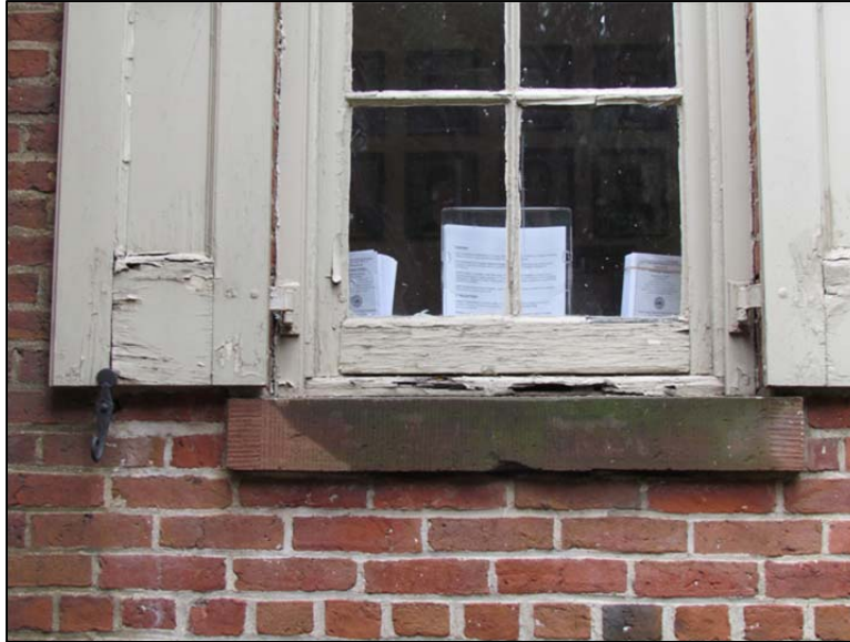
Figure 15: Arrows point to wood rot on the sill of window 111.
