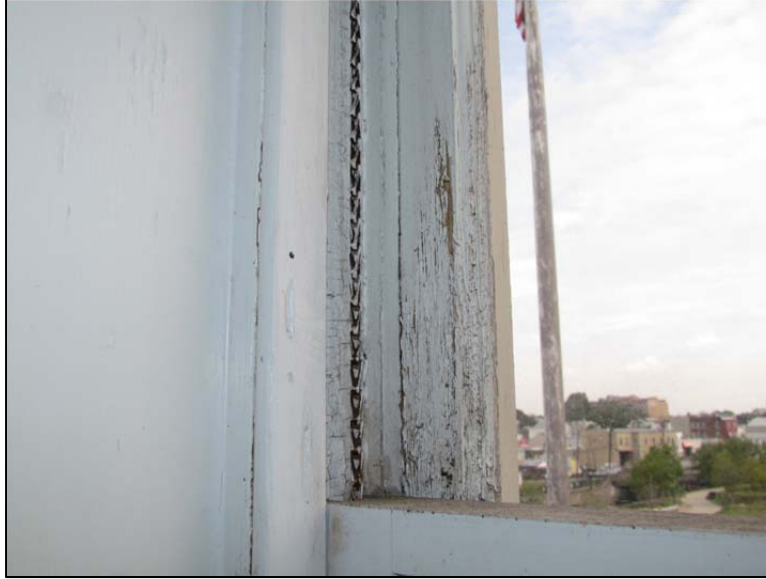
Figure 9: Wood deterioration to the stile of the upper sash of window 108.
