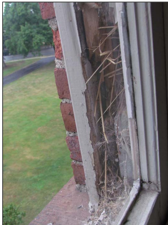
Figure 16: Extensive wood deterioration of the frame of window 308.
