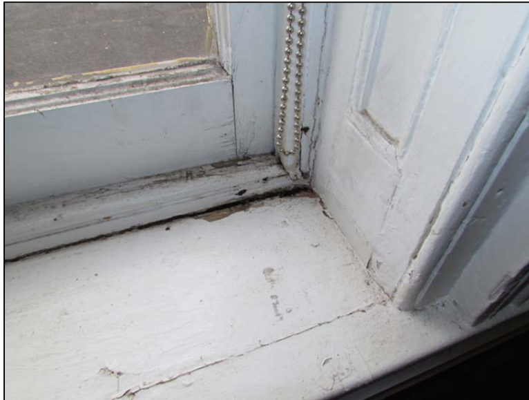
Figure 10: Wood deterioration on the sill of window 105.
