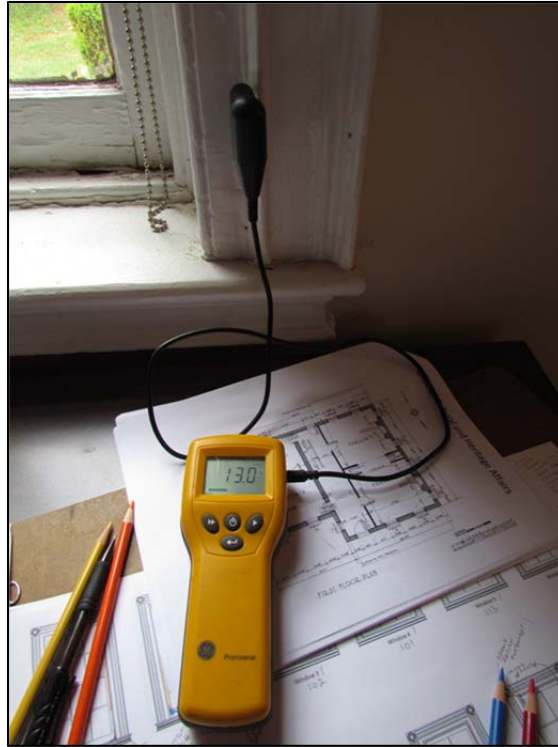
Figure 7: High percentage of moisture content in the wood of window 111.
