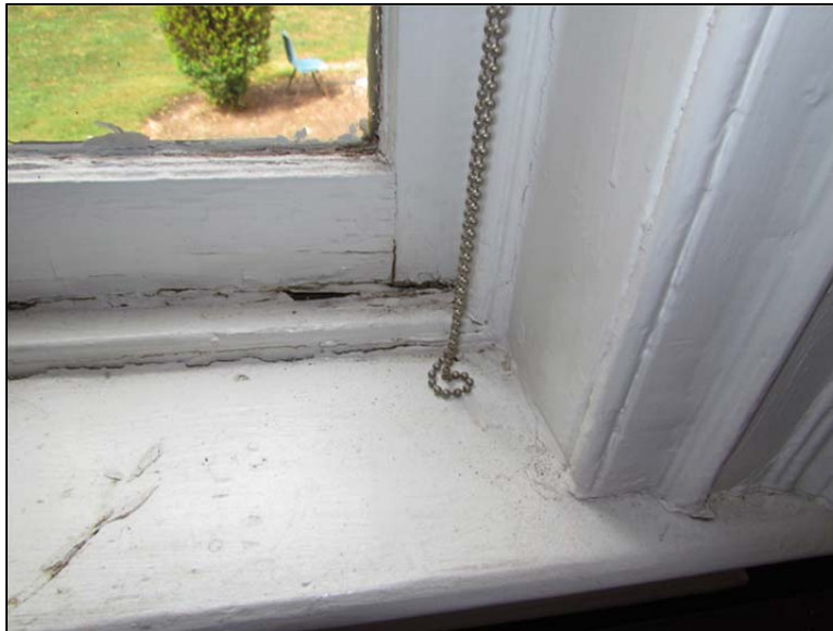
Figure 2: Typical condition of lower window sashes and sills as seen on window 111.
