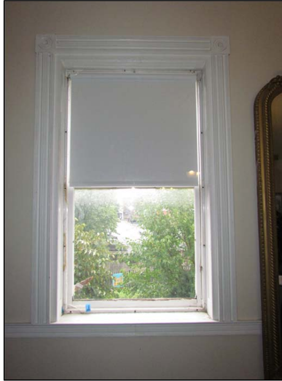
Figure 11: Window 103 which had its lower sash destroyed by Sandy.
