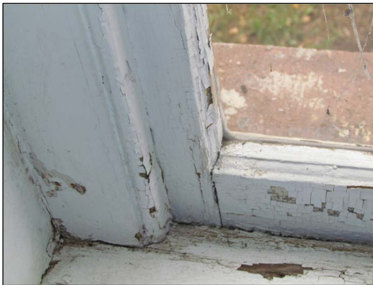
Figure 4: Paint loss on the bottom rail of window 101.
