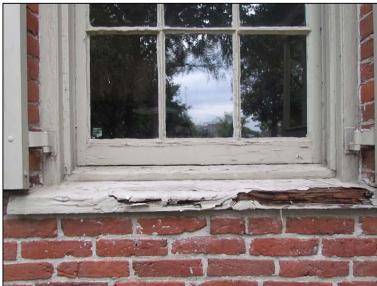
Figure 14: Extensive wood rot on the sill to window 112.
