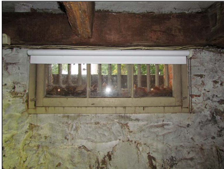
Figure 8: Water staining is seen on the wood of window B9.
