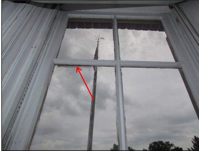
Figure 1: Arrow points to small area of remaining glazing putty on window 106.
