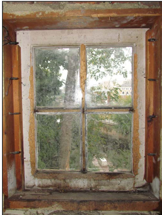
Figure 12: Wood of sash and muntins has been damaged by squirrels.
