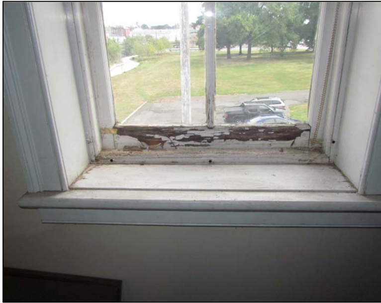
Figure 13: Extensive wood rot along the bottom rail of window 108.
