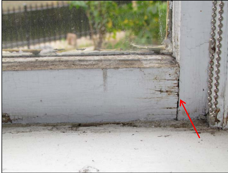
Figure 3: Arrow points to open joint at the bottom of the sash as seen on window 101.
