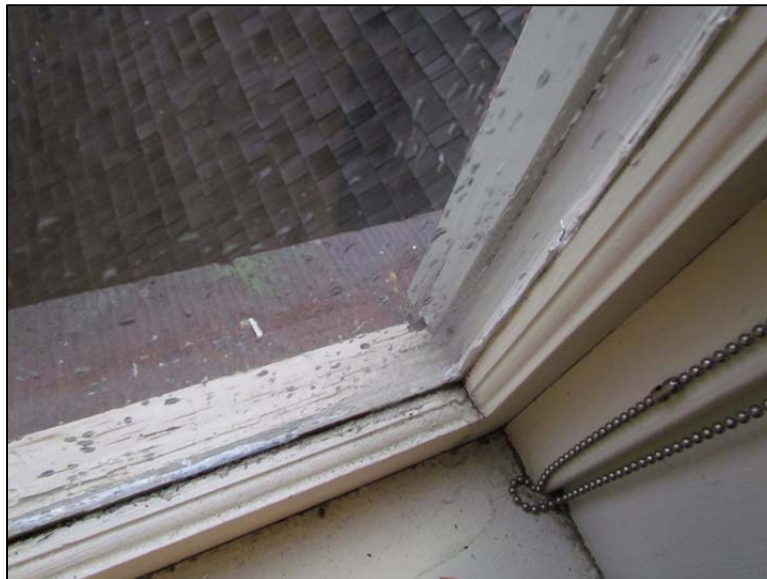
Figure 18: Typical condition of sill as seen on window 302.
