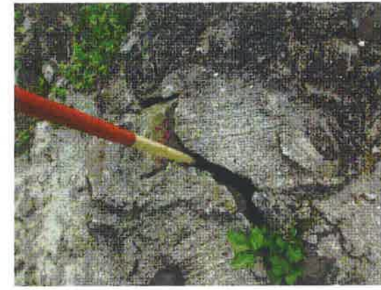
PHOTO OF CRACK TO BE REPAIRED BY ITEM ID
