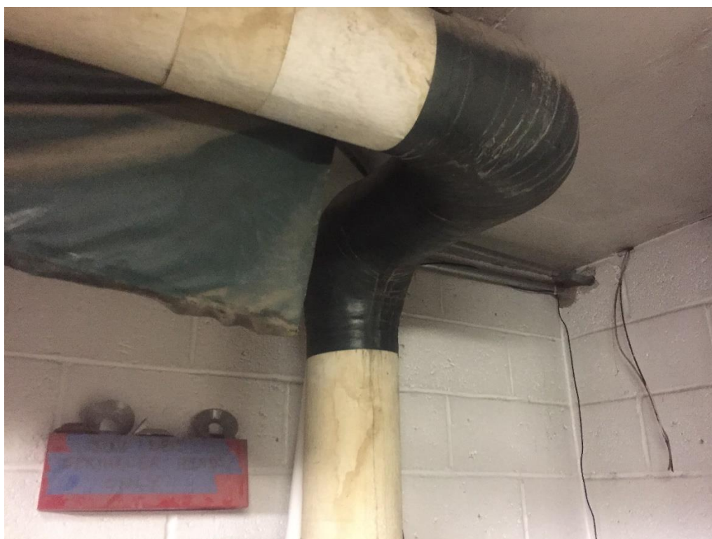
Sprinkler Room Fittings
