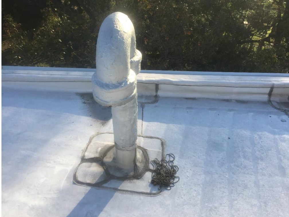
Drain Exhaust Vent
