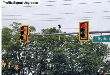
Traffic Signal Upgrades
