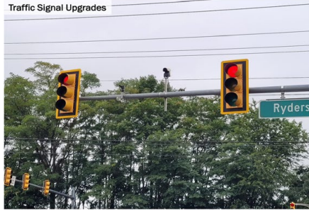
Traffic Signal Upgrades
