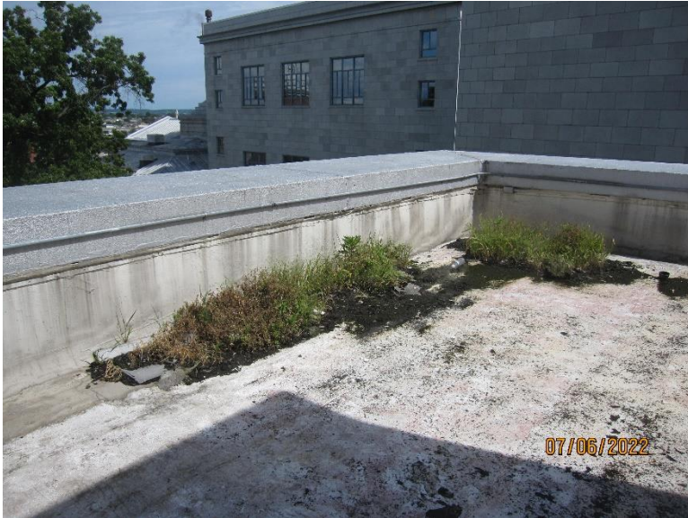
Photo 3- View of the Moss and vegetation is growing on the main roof.
