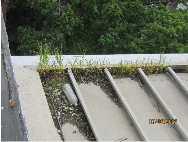
Photo 8 - View of the vegetation growing on the metal standing seam roof near the integral gutter.
