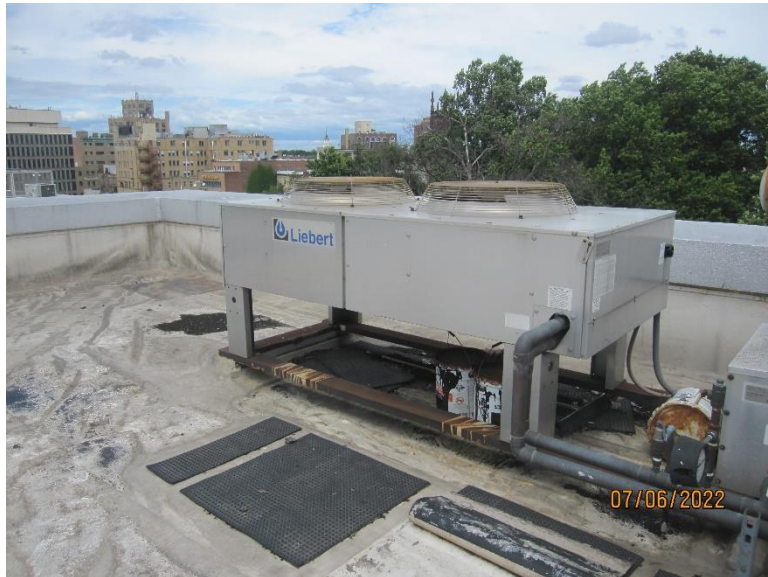
Photo 1 - View of the HVAC equipment located on the main roof. Note the equipment roof curbs on which the unit is located.
