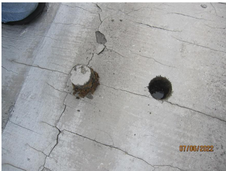
Photo 12 - Probe RP4 - View of the removed entirely saturated probe sample. Note the water filling within the hole where the removed probe was taken.
