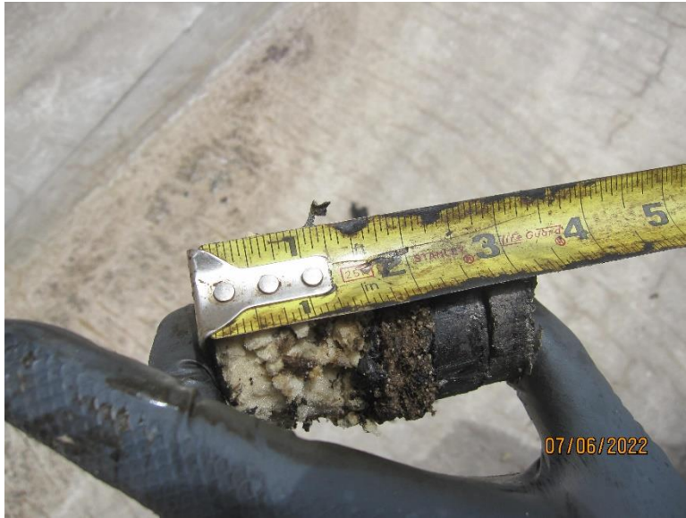
Photo 10- Probe RP2 - View of the removed probe sample. Note the saturated condition of the entire sample.
