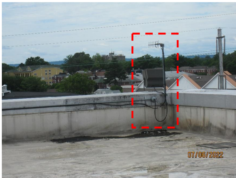
Photo 2 - View of the antenna attached to the parapet wall on the main roof.
