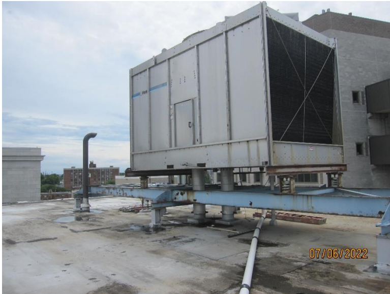
Photo 5- View of the large HVAC unit which is set on an elevated structural steel structure on the penthouse roof.
